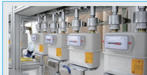
Remote meter reading
