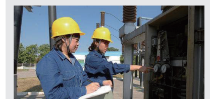
Power high temperature and high voltage monitoring
