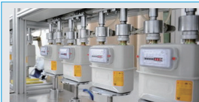
Remote meter reading
